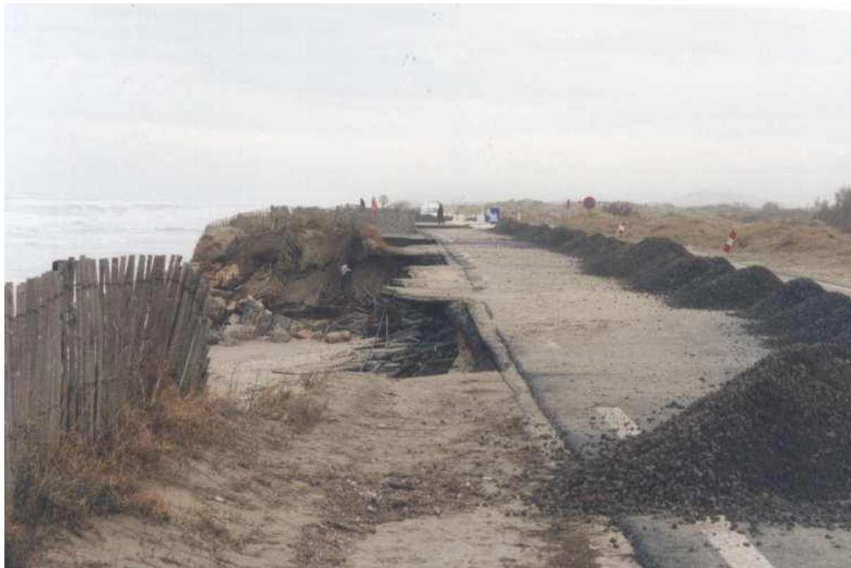
Pict. 1 : Recurent erosion impacts on the coastal road
