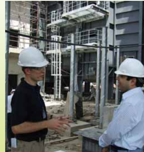
Engro Power Gen Ltd. – 200 MWe CCPP
