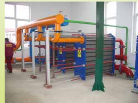
Oradea Geothermal Heating Plant
